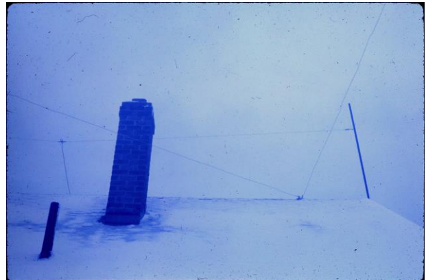
The WV2QPW Antenna Farm V-Beam Cause Roof Leaks Figure 2
