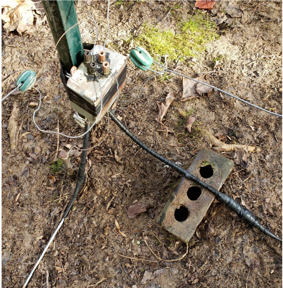
Figure 2. N4GG's K9AY Loop outdoor termination box.
