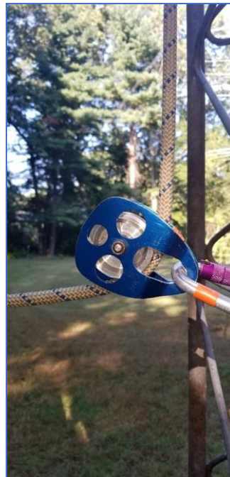
Figure 2. Use of a shackle and pulley to perform a 90 degree bend at the tower base. Courtesy of K1IR. This is a best practice.
