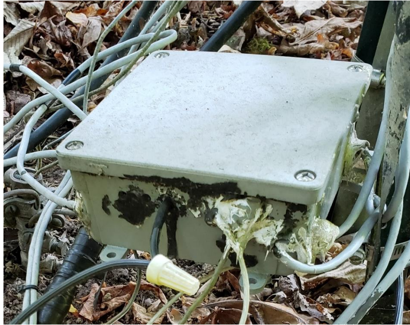
Figure 1. The outdoor junction box at N4GG – a rusty mess.
